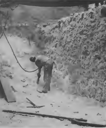
NO. 3, a boiler in operation at the No. 1 Powerhouse for 25 years, was shut down for the first time last month by Watertender Charles Hirsch (above). At the shut-down were (left to right) Fernando Eldige, assistant watertender, Arthur Lionberg, assistant fireman and Cyril Cayol, fireman. In front of the boiler a workman chips away at a hole which will house two boilers that will replace No. 3 and three other veteran steam producers.
